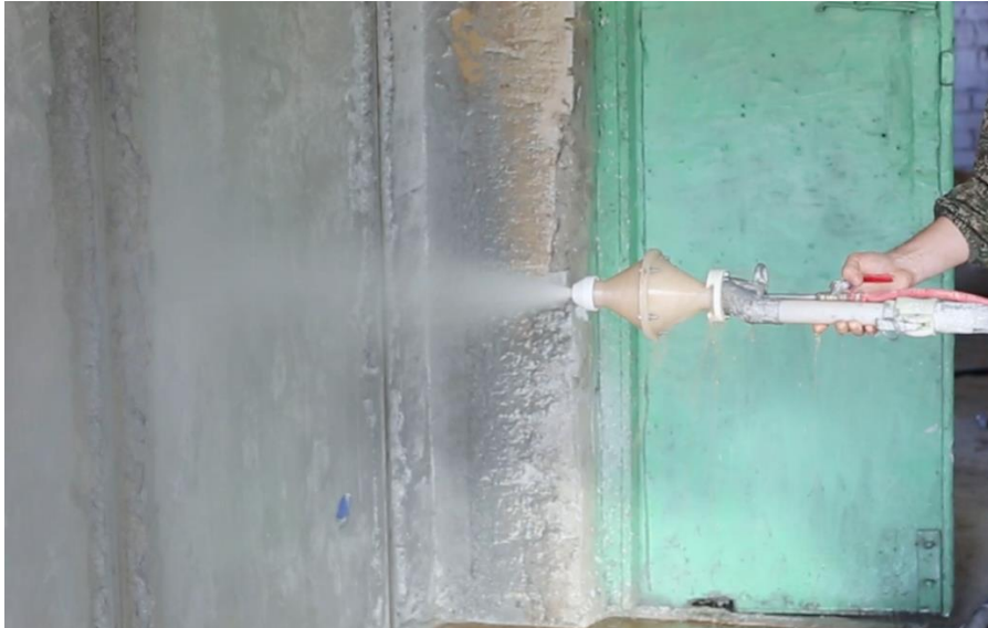
Fig.3. Application of the mortar using a nozzle for swirling the mixture onto a vertical surface
