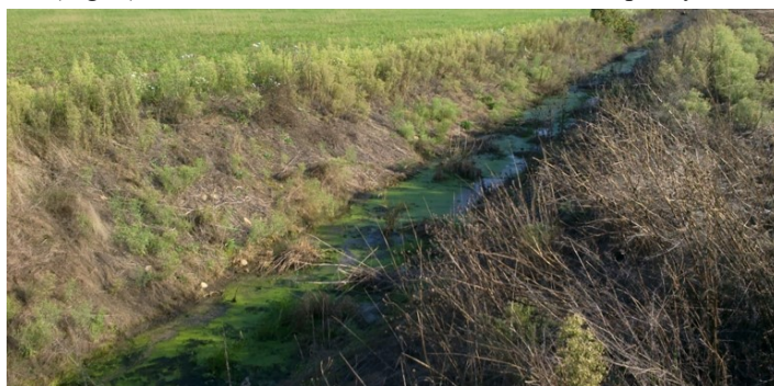
Fig. 1. Drainage canal condition during long-term operation without current and major repairs
