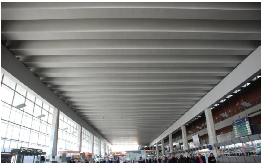
Fig. 2. General view of the load-bearing structures of the station building at the 1st floor level.
