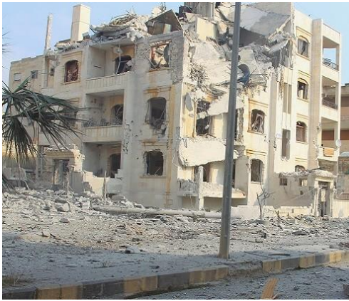
Fig. 5. Affected reinforced concrete building
