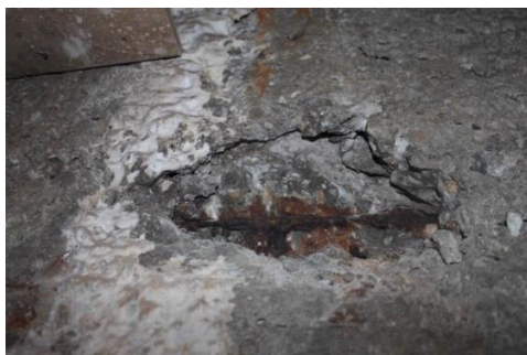
Fig. 3. Opening the bowl structure from the side to determine the existing pool bowl reinforcement state.
