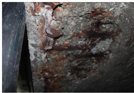
Fig. 4. Opening the structure of the pool bowl from the bottom side to determine the existing reinforcement state.
