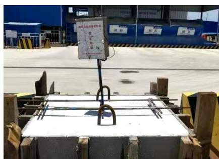
Fig. 2 Concrete temperature acquisition instrument
