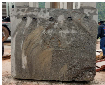
Figure 3 Cross-section photo of 11# bent cap cut across seam
