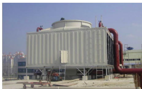
Figure 3. Low noise cooling tower
