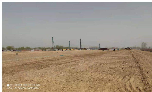
Picture 1 Settlement detection device
