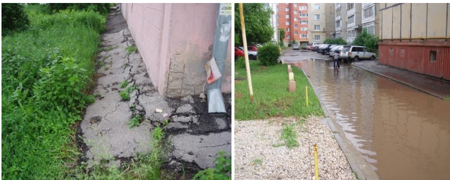
Fig. 4. Drainage system works unsatisfactorily, and the blind area around many houses is destroyed.
