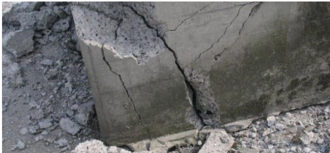
Fig. 4. Deformation of concrete by shear leading to slipping of the building.
