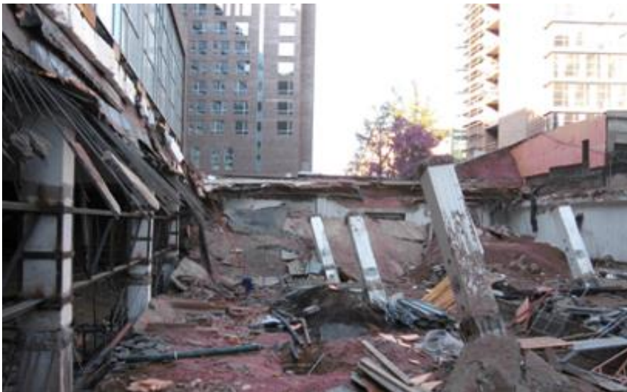
Fig. 1. Accident with successive collapse
