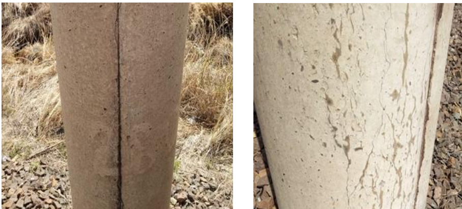
Fig. 4. Cracking of the support surface.
