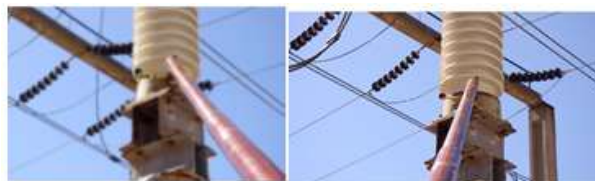
Fig. 2. Indicator on the support insulator in the 110 kV substation (Kazan TES-3).
