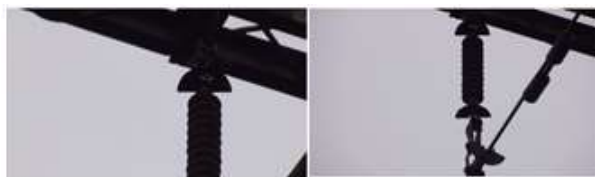
Fig. 3. Indicator on a suspension insulator 35 kV (Almetyevsk electrical networks).
