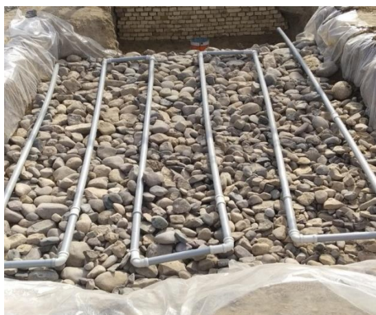
Fig. 3. Placement of heat pipelines in a helium greenhouse.
