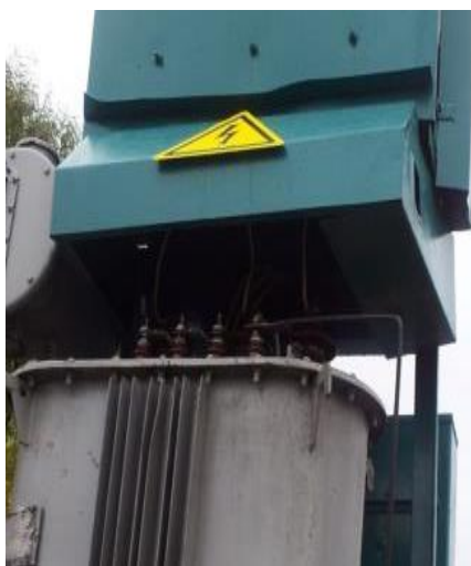
Fig. 1. Photo of the transformer housing installed at the 6-10 / 0.4 kV mast-type UTS of the branch of “IGDC of the Center” – “Orelenergo”.
