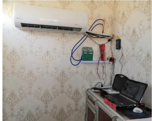
Fig. 3. Indoor unit with measuring devices, data recorder and laptop.
