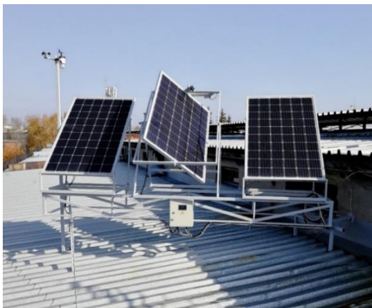
Fig. 1. General view of the main equipment of the experimental array
