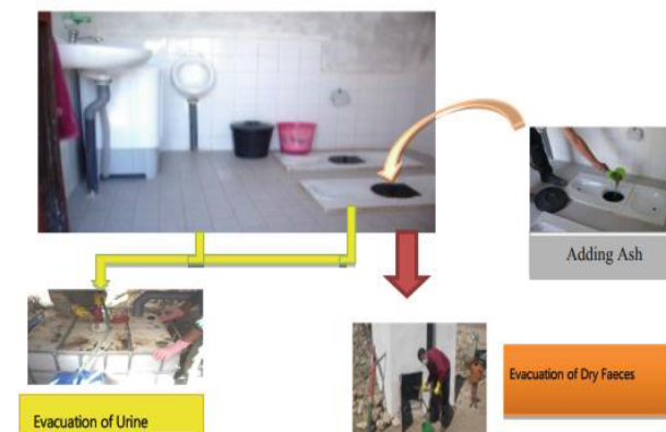
Fig. 2. UDDT installed at Dayet Ifrah Village
