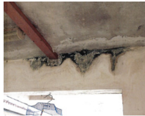
Fig. 6. Detection of moss due to water ponding.
