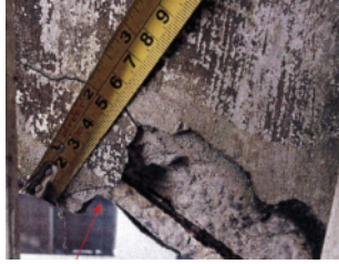
Fig. 4. Spalled soffit at third floor staircase of Block C.
