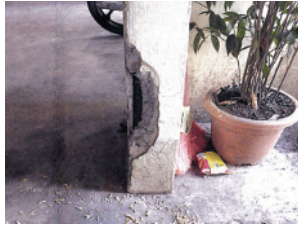
Fig. 5. Corrosion of exposed reinforcement system due to spalling of the column member at ground floor.
