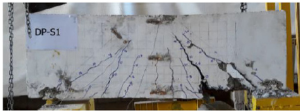
(a) Concrete cracking line of DP-S1-Exp.
