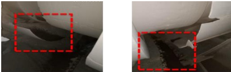
Fig. 3. Oil spill in the raw mill area before and after the installation of the Split-type oil seal
