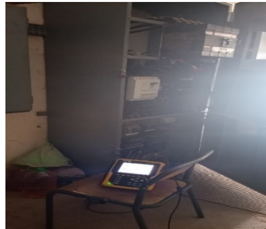
Fig. 1. Three-phase power analyzer recorder installed at the main circuit breaker
