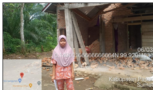
Fig. 12. Mr. Mardan's damaged house in Kajai, West Pasaman.
