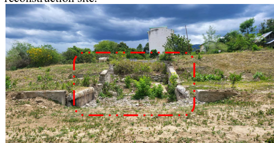
Fig. 1. The extensive damage in the Jono Oge irrigation canal.
