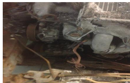
Fig. 4. A part of electrical wiring that comes from the generator.
