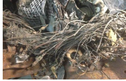
Fig. 2. Part of the electrical wiring of the motor harness.
