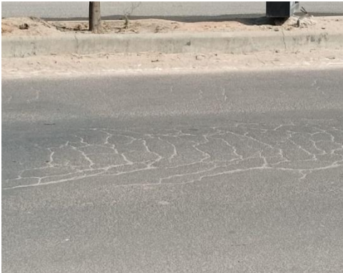
Figure. 5. Measuring of Cracks
