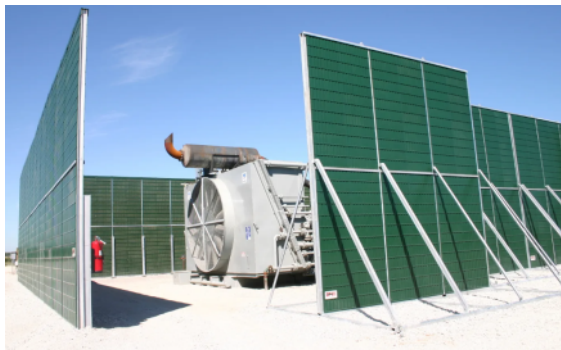
Fig. 3. Application of screens for noise protection during operation of crushing plants and dismantling equipment.
