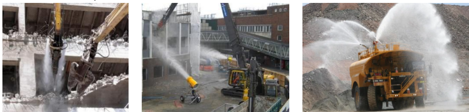
Fig. 2. Examples of water irrigation methods to reduce dust generation during demolition of buildings.
