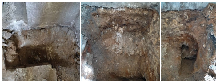
Fig. 1. View of the state of the foundation in the pit № 1, 2, 3.
