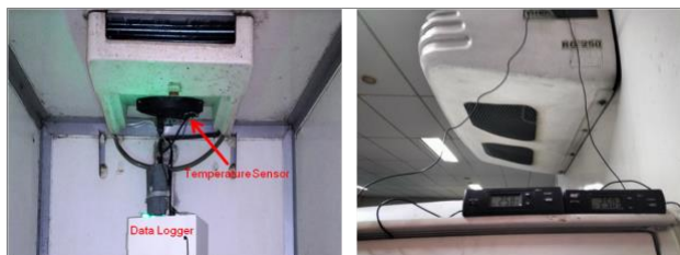
Fig. 1. Installation position of temperature sensor
