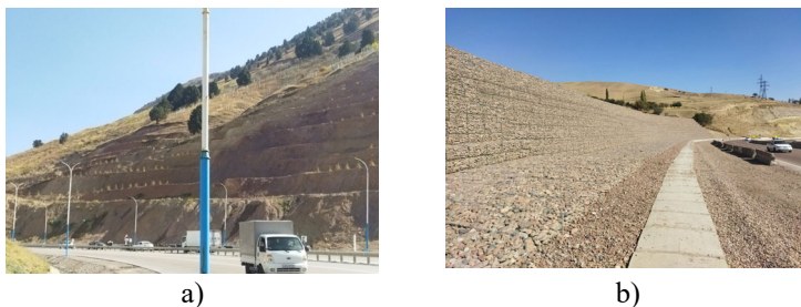
Fig. 4. Engineering solutions used to increase the stability of slopes against sliding in the “Kamchik” pass: a) construction of piles while reducing the frictional mass on the slope; b) use of gabion structure to prevent sliding on a loess slope (Source compiled by the authors).
