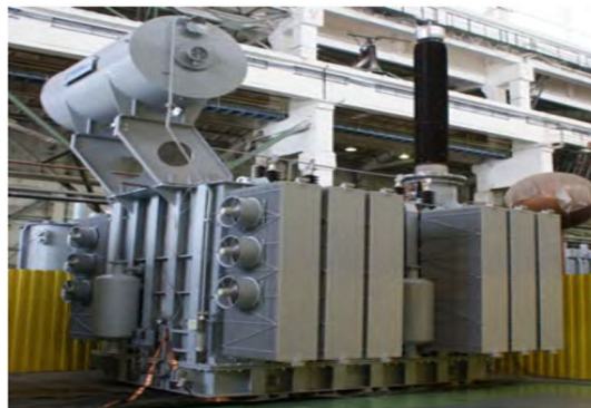
Fig. 6. Electromagnetic part of a 60 MVA controllably shunt reactor transformer with a voltage of 500 kV.
