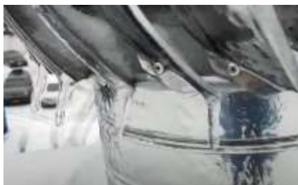
Fig. 8. Icing of the deflector of the natural ventilation system.
