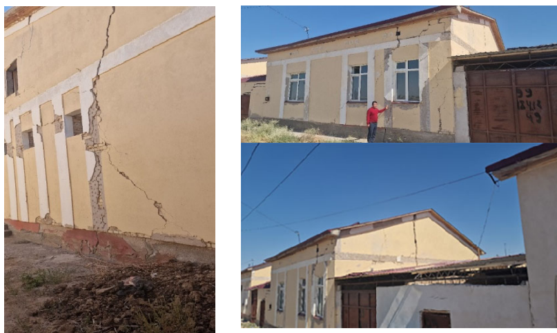
Fig. 2. The manifestation of cracking in buildings in the case when the foundation is completely in the zone of possible deformations.
