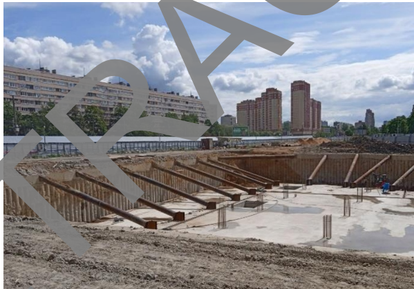
Fig. 8. The firing system installed on the binding belt of the foundation pit fence (using the example of the foundation section № 3)
