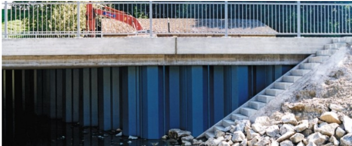
Fig. 4. View of abutment consisting of steel sheet pile LARSEN 703 SP on a bridge with a 7m span.
