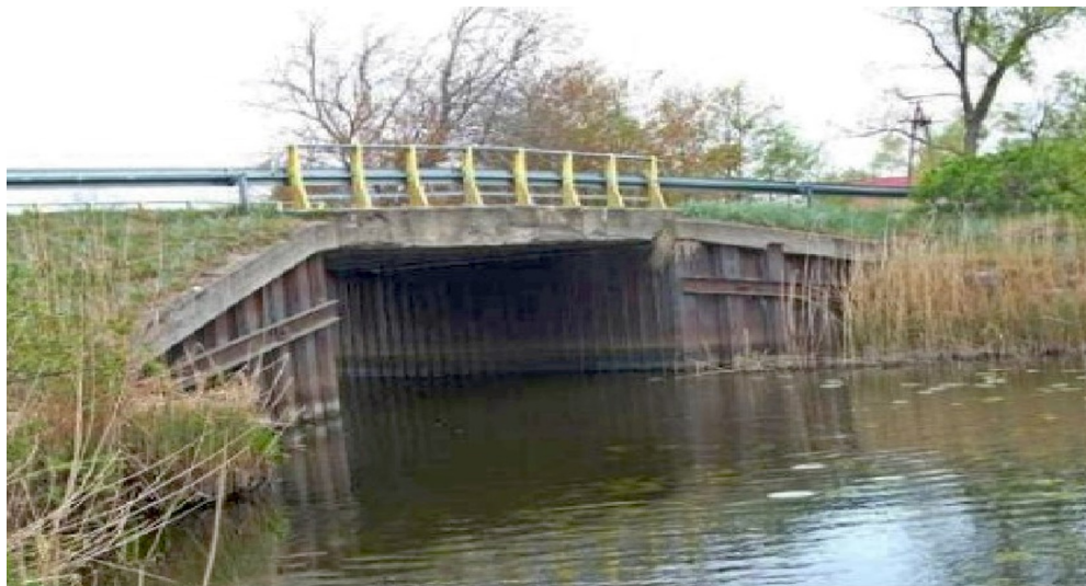
Fig. 6. Bridge with integral abutments - sheet pile walls from the beginning of the 20th century.
