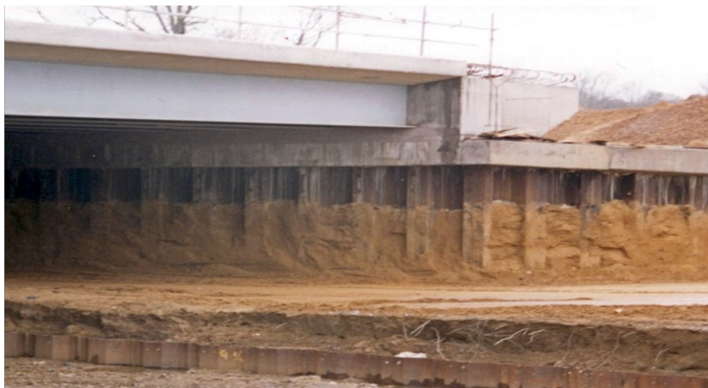
Fig. 2. Bridge with integral abutments consisting of steel sheet pile walls and a steel-reinforced concrete connecting beam.
