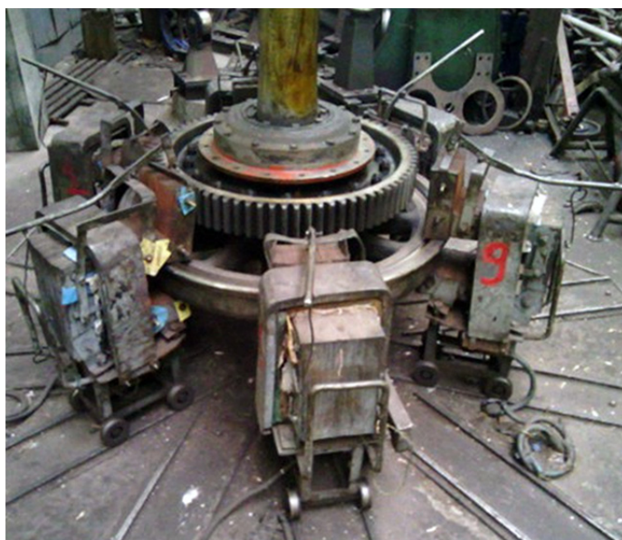
Fig. 1. General view of an induction heater with a wheelset installed for heating the bandage bracelet.
