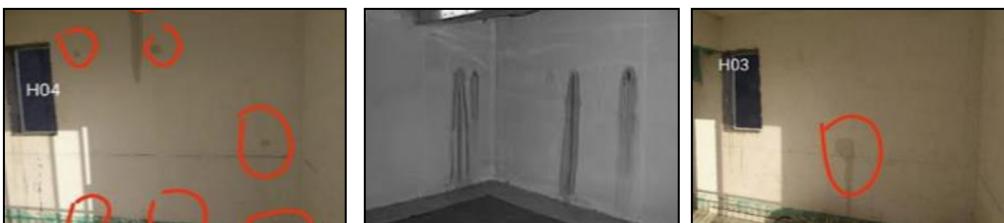
Fig. 3 External Wall Leakages
