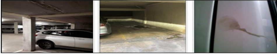
Fig. 7 Water leakage through car parking roof
