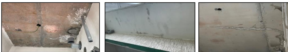
Fig. 6 Leakages through Toilets and Bathrooms
