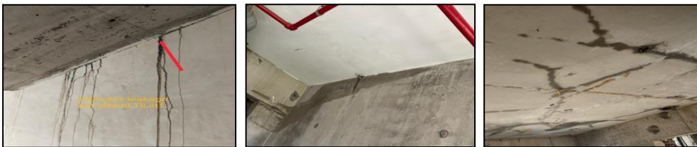
Fig. 2 Terrace and Roof Leakages
