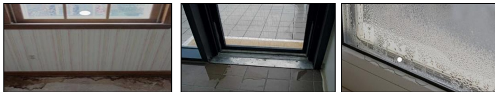
Fig. 5 External Window Leakages
