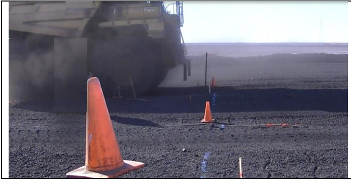
Fig. 9. Road surface with evident deflection and cracks under the load of a moving 100-ton haul truck
