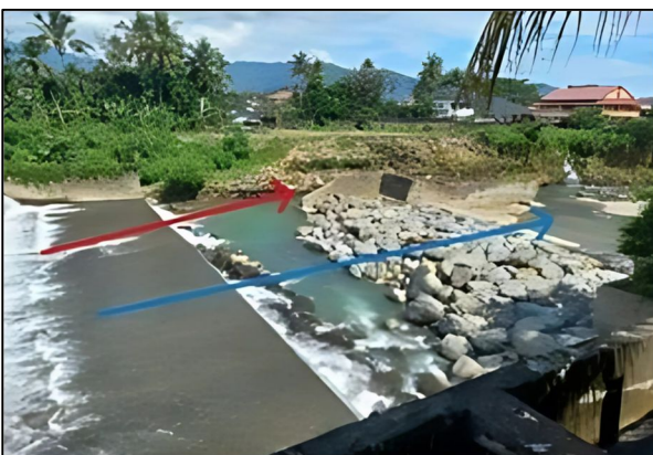
Fig. 4. Concrete turret not working
