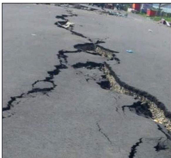
Fig. 3. Tensile cracks arising from lateral spread in the Siteba residential area [3].
