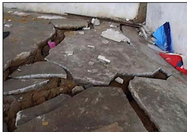
Fig. 4. Uplifted floor slabs in the residential area of Perumdam, Padang City [3].
