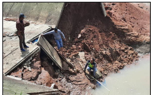
Fig. 1. The primary canal in the North-Raman irrigation-area collapsed
