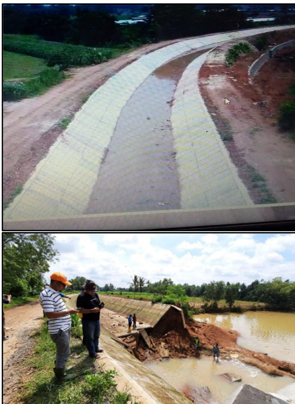
Fig. 7. The primary canal: before landslide (top) and after landslide (bottom).
