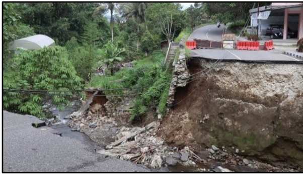
Fig. 2. Infrastructure damaged by flash floods following the eruption of Mount Marapi in West Sumatra
