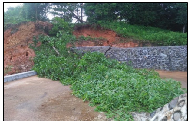
Fig. 1. Damage to gravity walls
