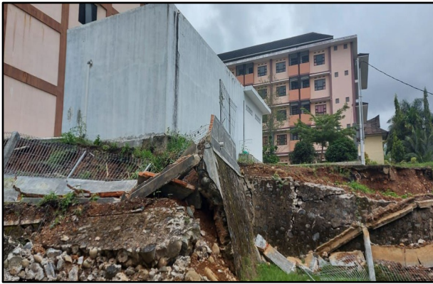
Fig. 2. Damage to gravity walls in student dormitories
