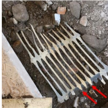
Fig 8. Large scale test sample following excavation. Arrows show location of connector damage.
