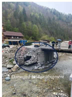
Fig. 1. Damaged Bridge abutment in the municipality of Črna na Koroškem, Slovenia (2023)
