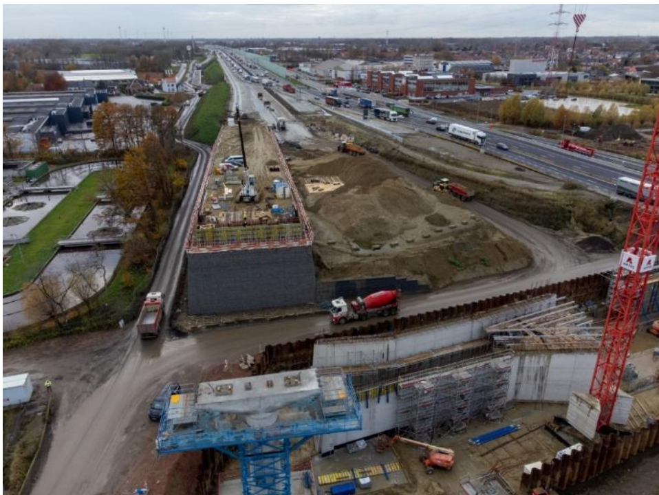
Fig. 2. Reinforced fill structure to be connected to the road supported by a reinforced concrete structure on pillars.
