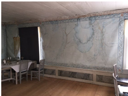
Fig. 2. Festivities room in Erik-Anders Farm, showing significant moisture «blooms» on the southwest exterior wall.
