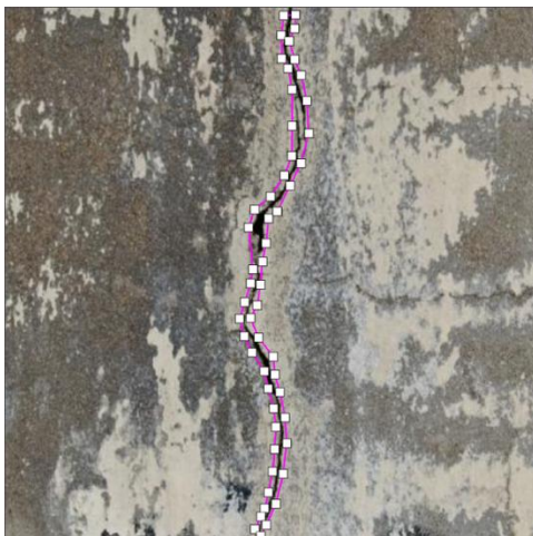
Fig.3. Annotated vertical cracks on the surface of concrete
