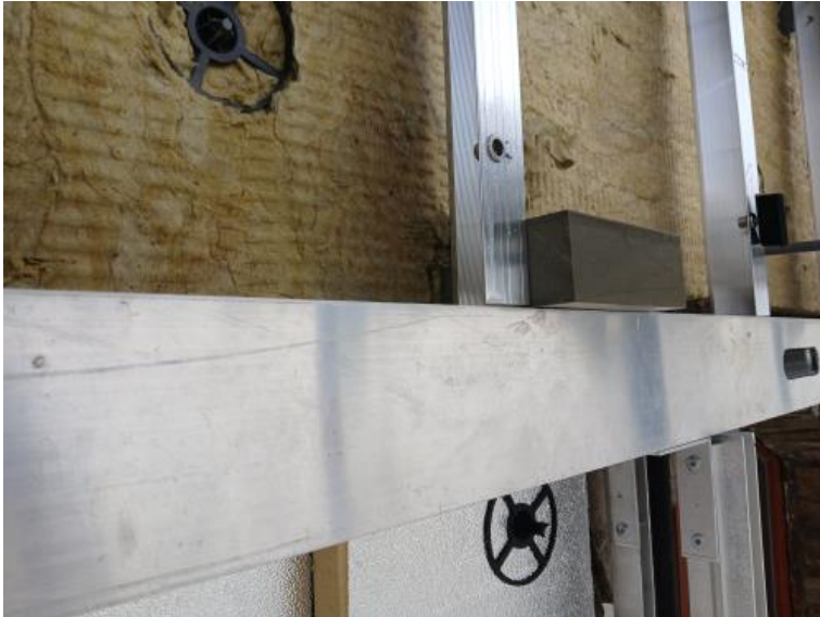
Fig. 6. ADBE structure fixed to the wall.
