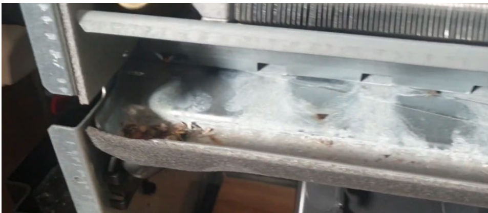
Fig. 1. Illustrative non-exhaustive picture of drain pan of a fan coil unit which collecting water as condensate from the cooling coil, may become a place where also dust and particulate can be collected. The mixture of condensed water, dust and particulate can potentially create good conditions for bacteria proliferation.
